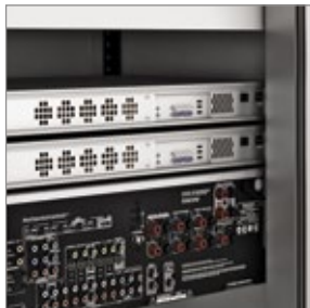
Storage cabinets with rack mounted A/V equipment
